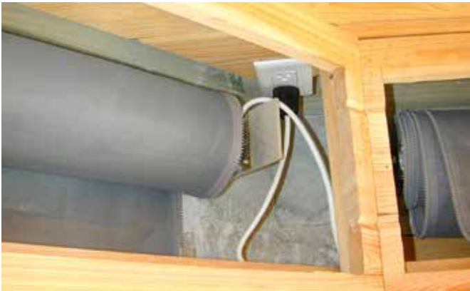
Duplex electrical outlet installed inside the cavity outside the working area of the screen roller, mesh and motor.
