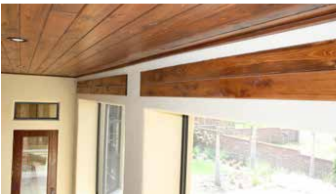
Removable front access panels finished to complement wooden tongue and groove ceiling.
