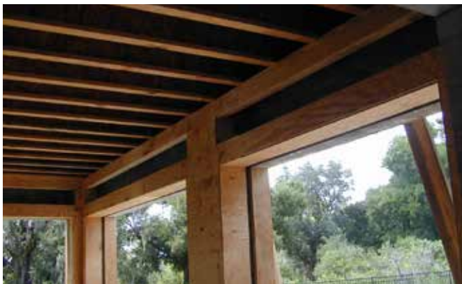
Cavity framed in top of header opening with front access. U-channel mounted in columns surrounded by framing before stucco finish is applied
