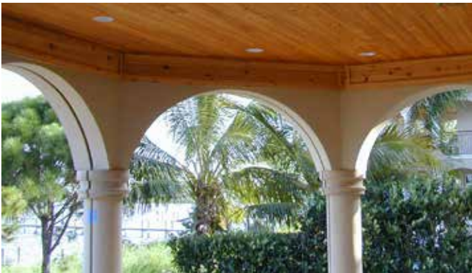
Motorized screens recessed within multiple arched openings, with removable front access panels.
