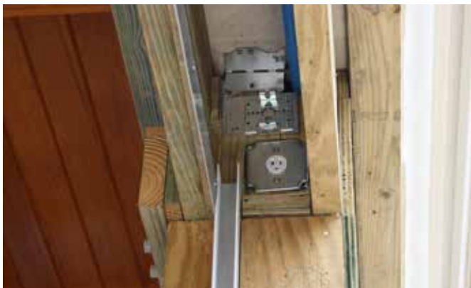
Unfinished cavity and column showing mounting brackets, electrical connections, and u-channel placement.
