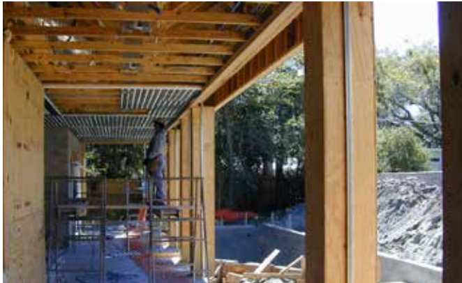
Cavity framed in top of opening with bottom access, u-channel mounted on column before finish is applied.
